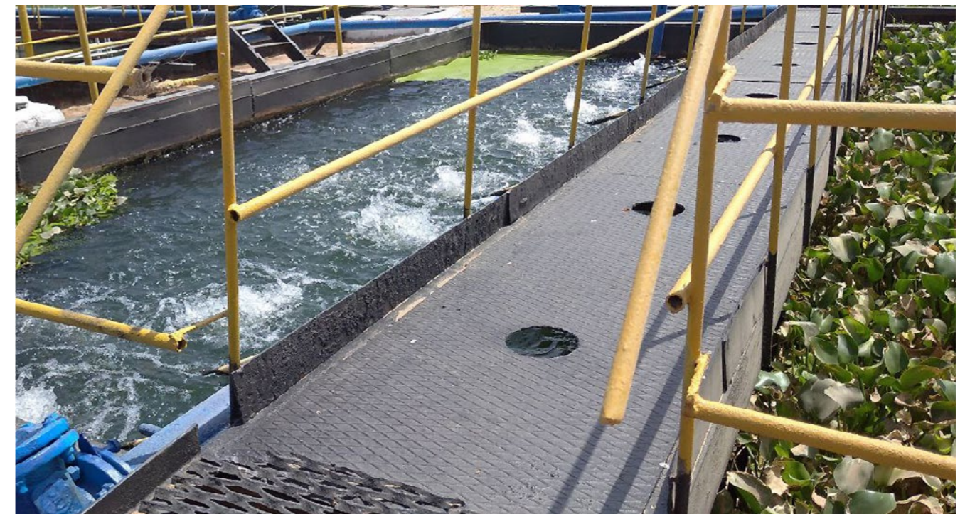
Clearing treatment of domestic wastewater with Eichhornia and Pistia plants at the Mubarek Gas Processing Plant
